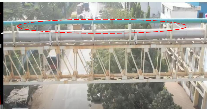
Nitrogen Pipeline Network
