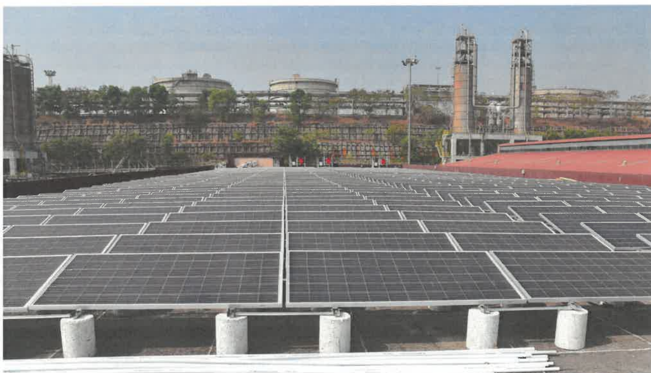
MRPL Solar unit inside the refinery
