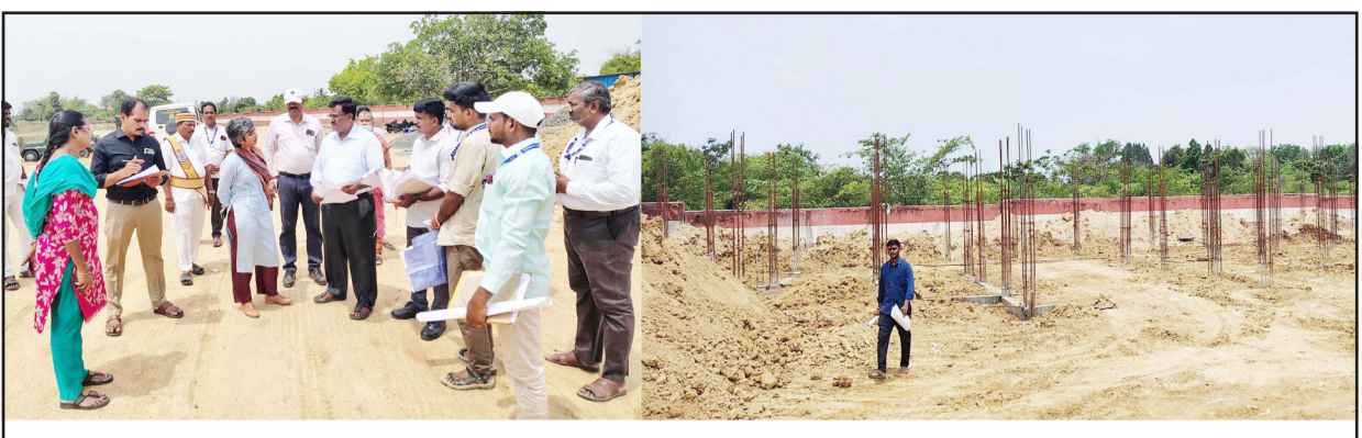
Kanchipuram Collector T. Sneha inspected the construction of a Regional Transport Office with a test track, being built at a cost of Rs.7 crore near Vadamangalam Ooratchi Koot Road in Sriperumbudur. Thirupurur Revenue Divisional Officer C. Balaji and Public Works Department Executive Engineer Somasundar are also present.
