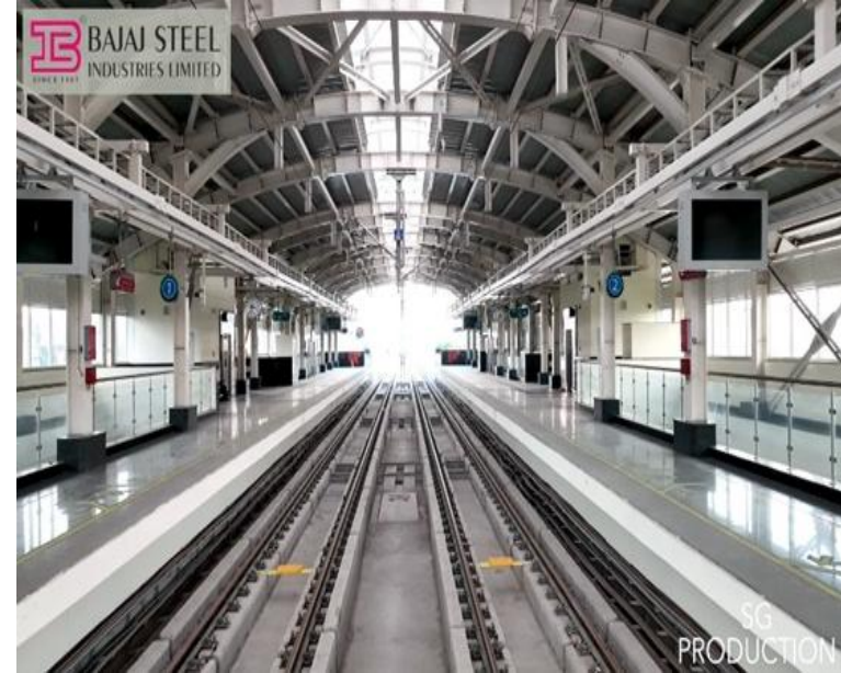
Metro Station, Nagpur – Fire Fighting System
