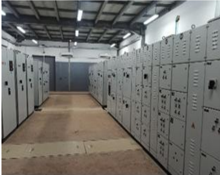
Electrical panel supplied to one of our Foreign Client
