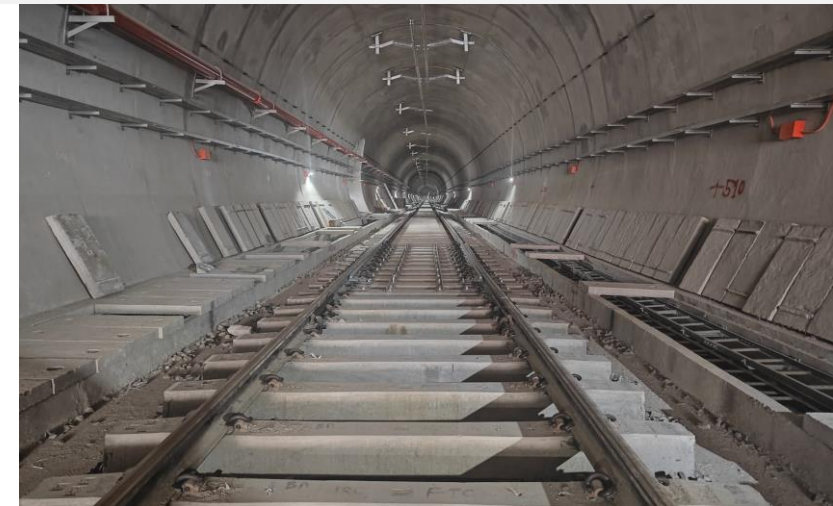
Tunnel Ventilation project, West Bengal
