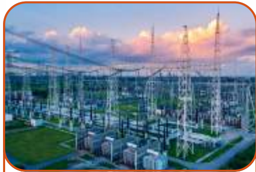
Power & Electrical Infrastructure
