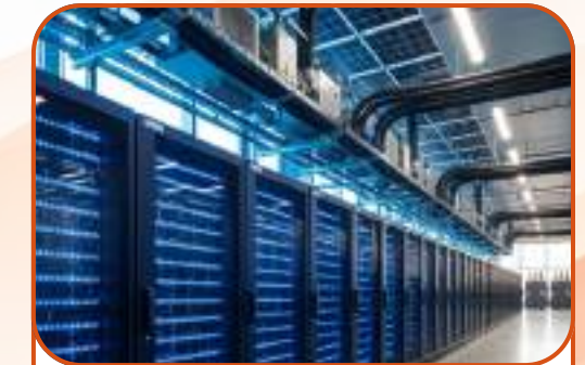
AI & Data Centre Infrastructure
