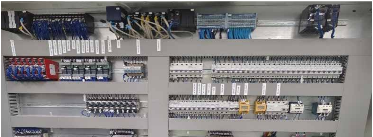
Panel with RCCB & overcurrent protection
