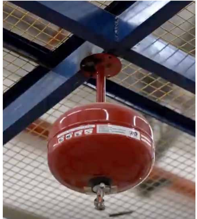
Advanced fire systems
