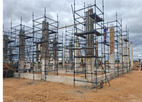
400kV Mmamabula Substation project (Botswana)
