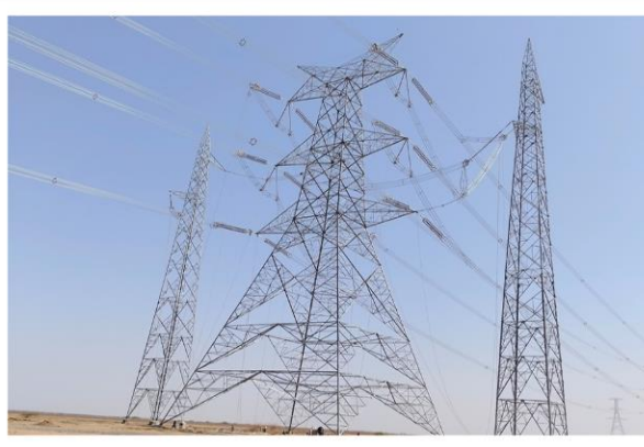
765 kV D/C Transmission lines in Khavda, Gujarat
