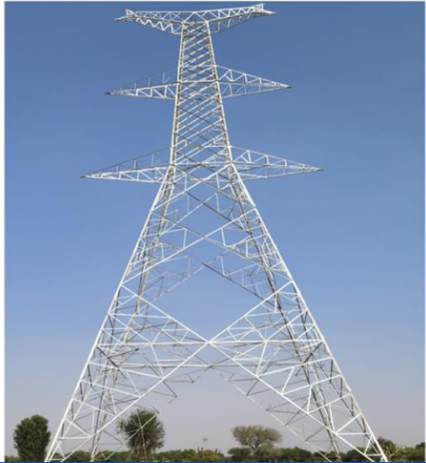
Koppal-II PS – Narendra (New) 765 kV D/C line
