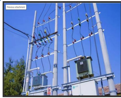
EPC RDSS (Revamp Distribution Sector Scheme)
