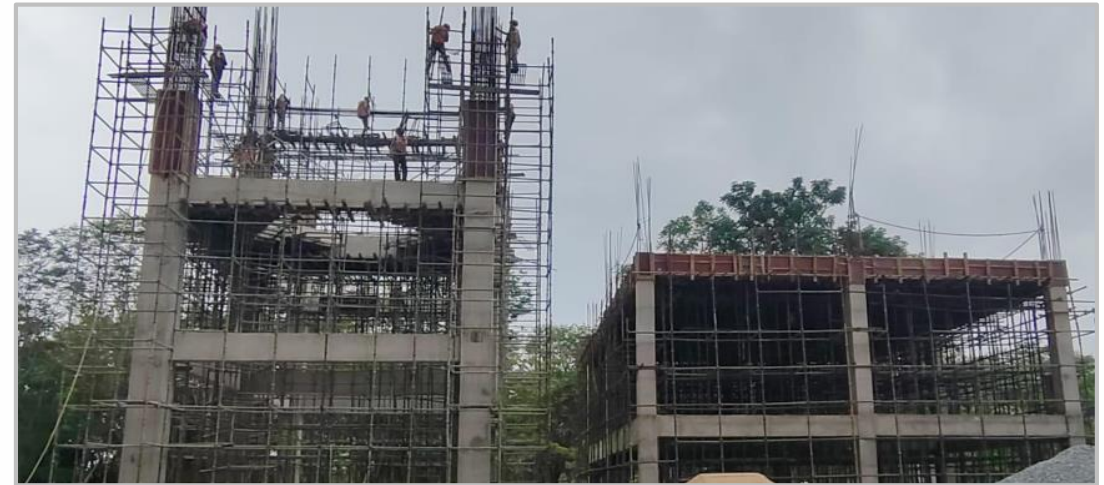
Nandyal IU: Chlorine Bypass - Baghouse and MCC Room
