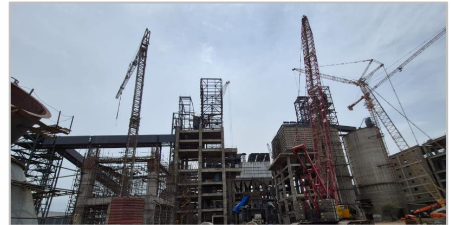
Nagaur IU – Cement Grinding and Packing & Dispatch
