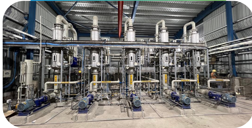
Waste Heat Evaporators
