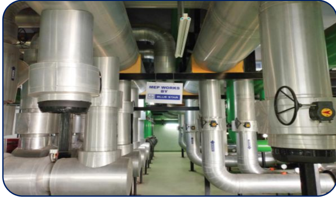
Electro-Mechanical Projects and Commercial Air Conditioning Systems
