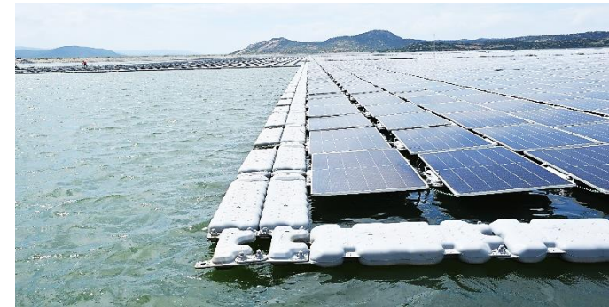
20MW Floating Solar Project at Vijayanagar, Karnataka
