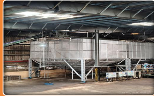
Silos for holding, drying, and batch-wise weighing of RCN
