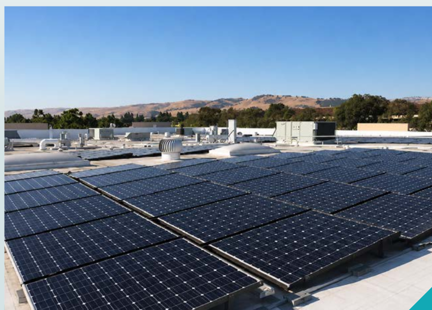
Utility industrial solar mounting structures
