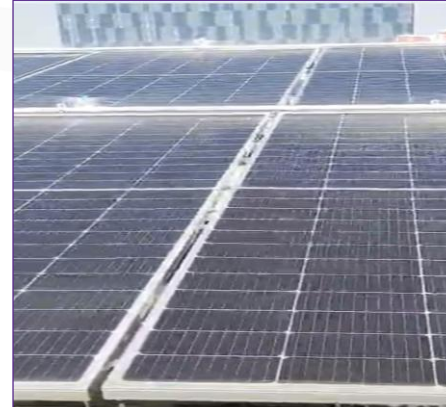
Rooftop solar installations
