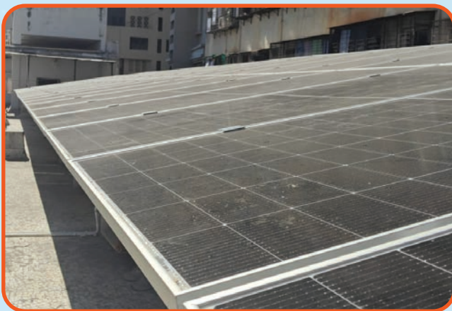
Installed 50Kw Rooftop On-Grid Power Plant System at Brihanmumbai Municipal Corporation, Maharashtra
