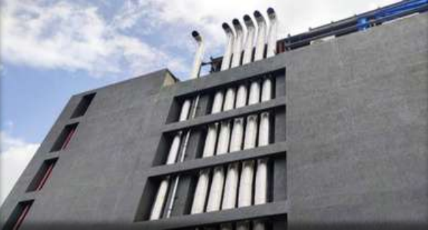
DG Platform & Exhaust System
