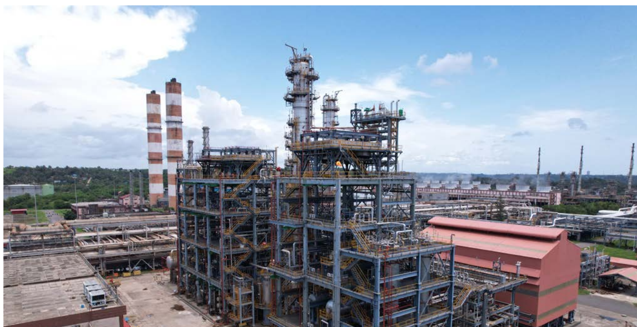
FCC Gasoline Treating Unit
