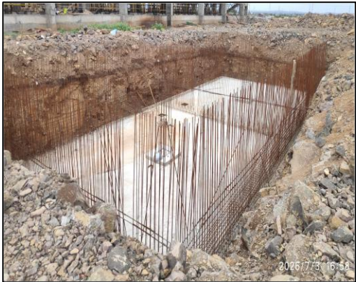
Raw Water Tank
