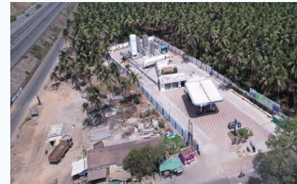
LNG/LCNG fuel stations
