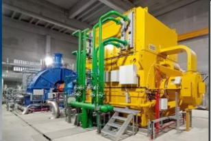
Steam Turbine Generator & Site Installation
