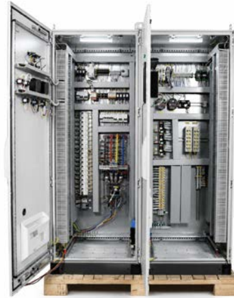
Distribution & automation panel
