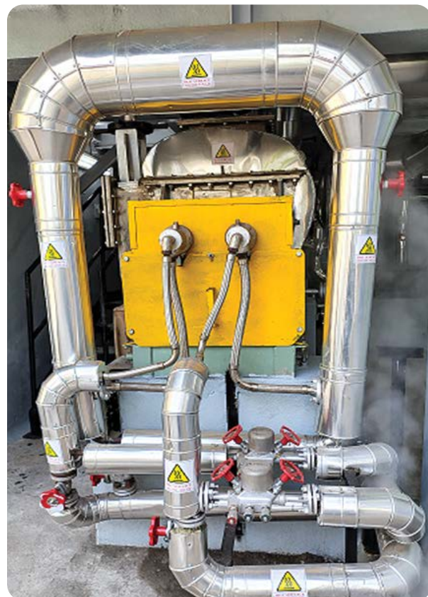
■ Sludge Dryer, Pithampur
