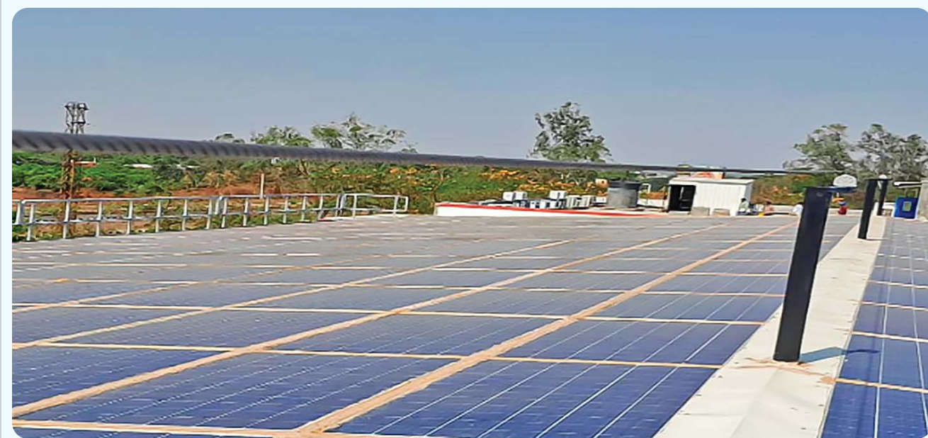
Solar Panel at Digwal, India
