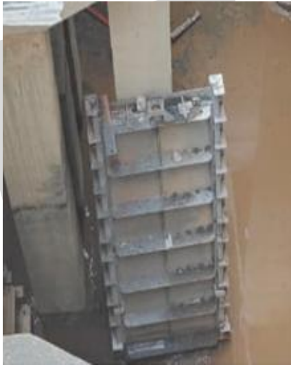
Multiple Size Gates & Screen for 400 MLD Desalination Plant Chennai
